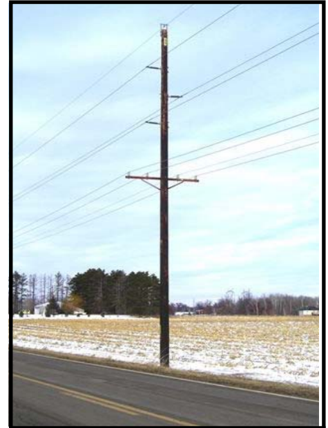
Typical 69 kV Transmission Line With Distribution Underbuild
